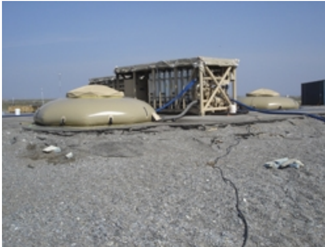
The EUWP ultrafiltration unit and two water transfer tanks at Port Clarence, Alaska.
