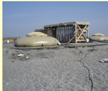
The EUWP ultrafiltration unit and two water tanks at Port Clarence, Alaska.
